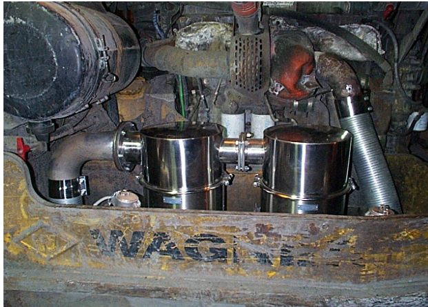
Figure 2: SiC DPF installed on LHD
