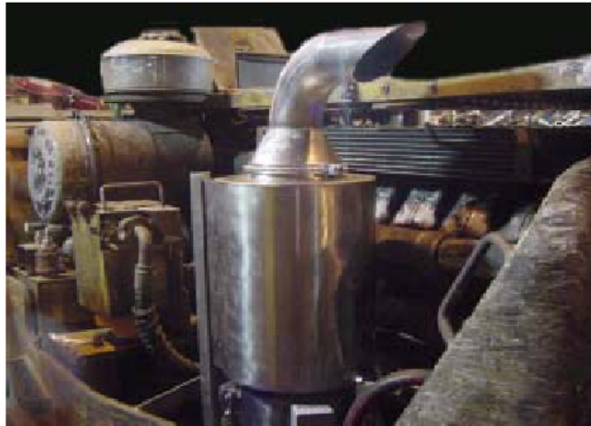
Figure 3: SiC DPF installed on LHD
